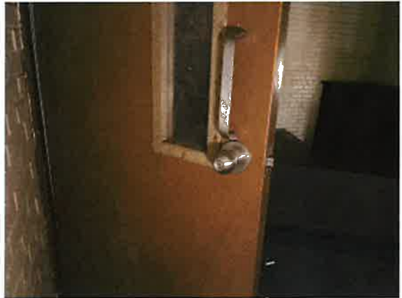
Photo 6 LCP, locker room door paint
