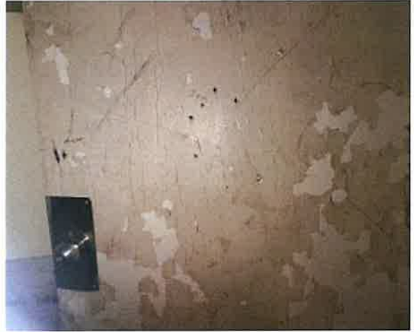
Photo 4 LCP, locker room door paint
