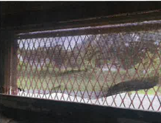
Photo 5 LCP, window paint
