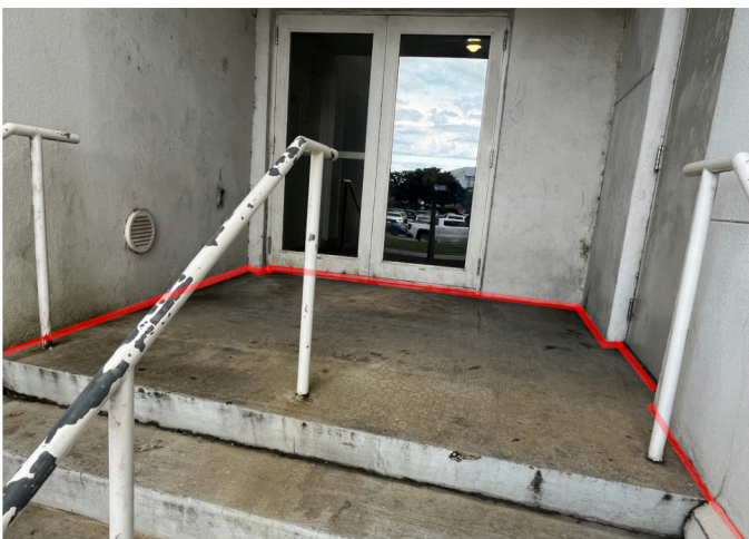
2. Large stairwell leading to Exploreum along Water Street
