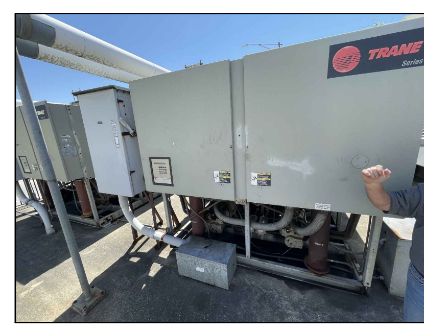
DISCONNECT FOR CHILLER #2 TO BE REMOVED AND REPLACED NEW
